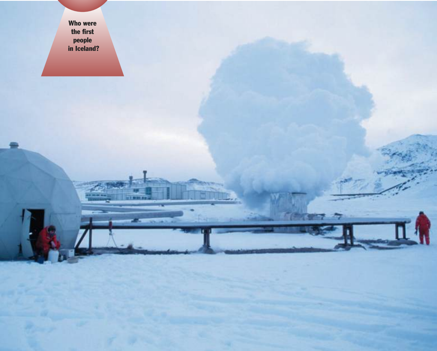
This power plant produces heat for the city of Reykjavik using steam from hot springs.
